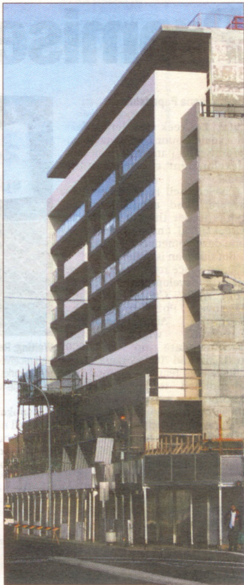
Up and up: Construction is under way for a nine-storey building by Veeco Holdings in Bay Street, Brighton-Le-Sands. Picture: Chris Lane
